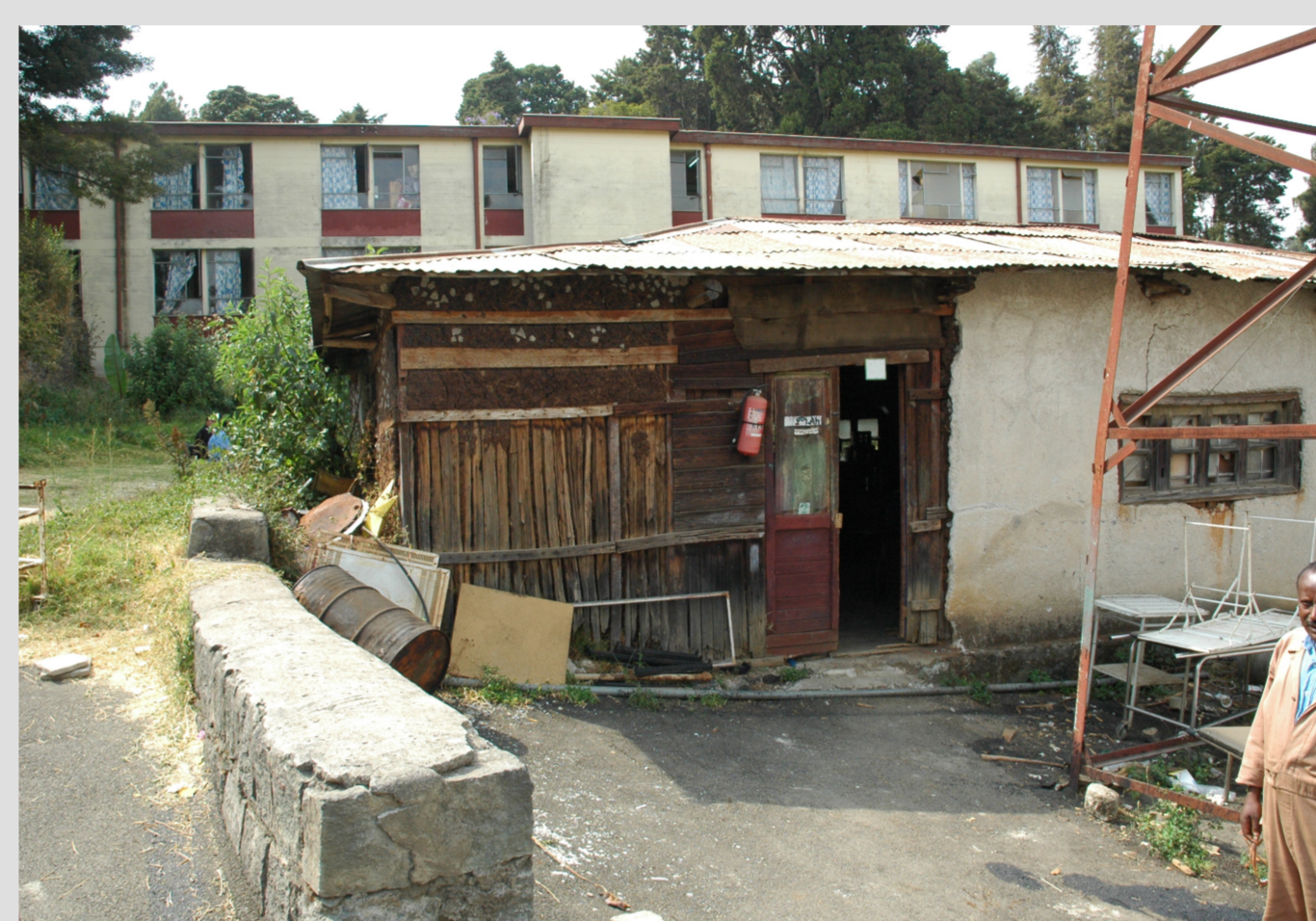
Fig 4: This medical equipment workshop at an African hospital illustrates the low priority given to the upkeep of medical technology assets in many developing countries
