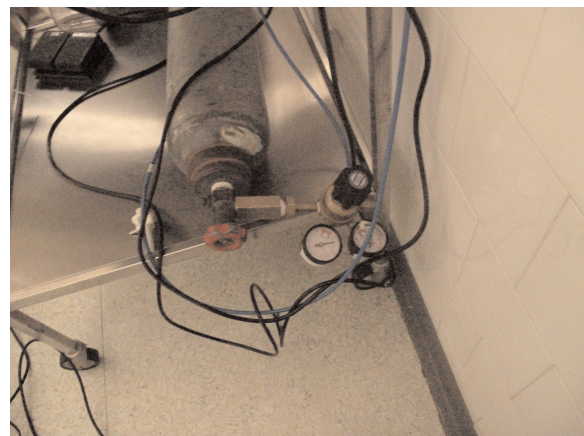
Incorrect storage of a cylinder
